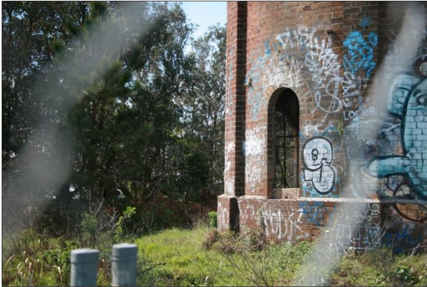
Figure 98: Deterioration to the building is also noted to the brick tower, note the missing sill to the arched opening. Weir Phillips
