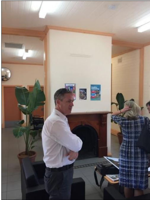
Figure 72: Waiting room interior with central fireplace. Note the timber lined walls and later floor tiles. Weir Phillips
