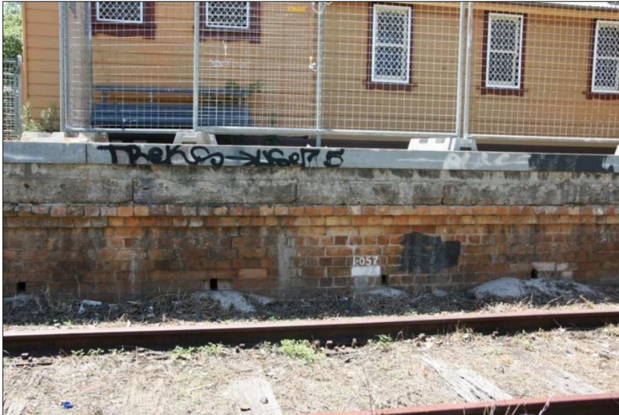
Figure 113: Detail of platform edge showing brick wall set beneath concrete slabs and topped with metal trim. Weir Phillips
