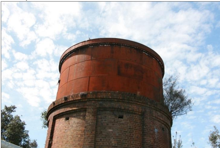
Figure 97 The tank is deteriorating. The corrosion has formed holes beneath the upper rim. Weir Phillips
