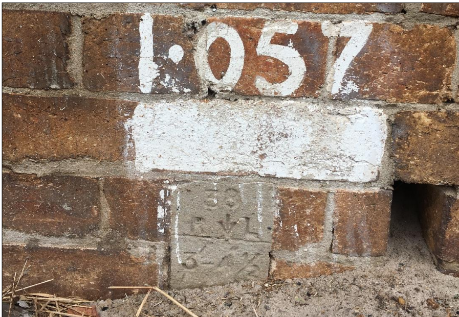
Figure 114: The platform face includes details such as the survey marks believed to date from the construction of the platform. Plummer and Smith
