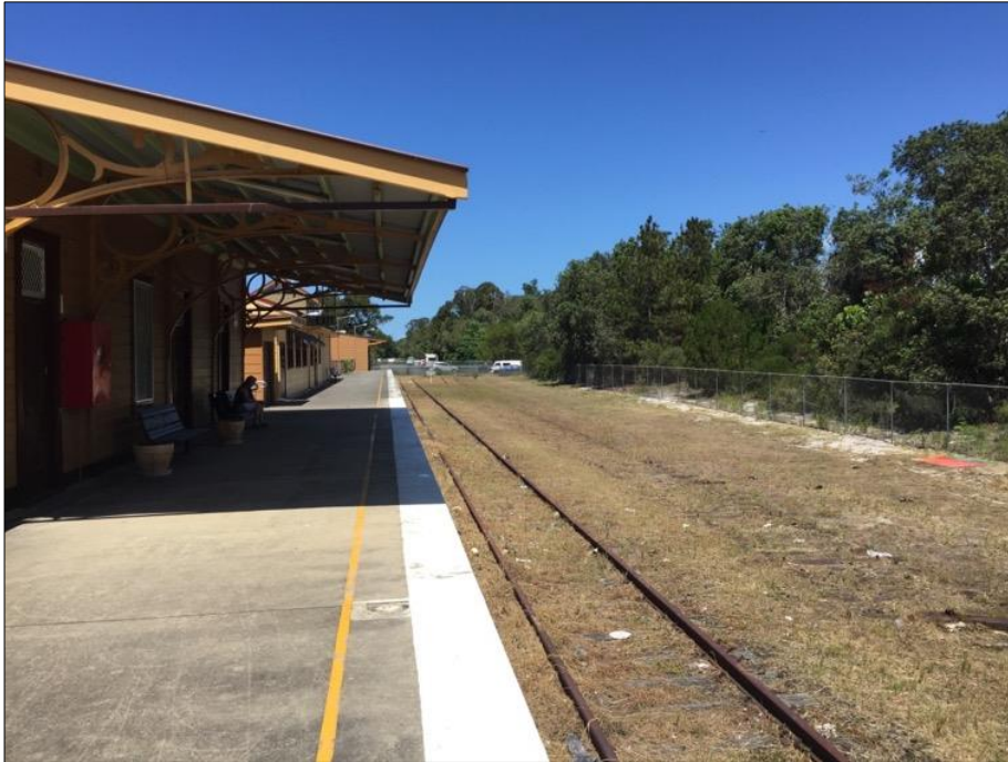
Figure 69: Photograph showing the platform and the former railway track and track bed. Also visible is the perimeter fence addition.
