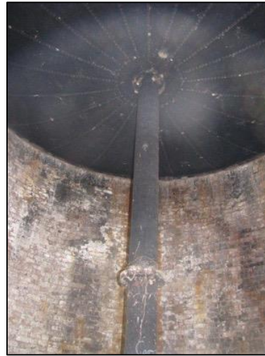
Figure 122: Interior of Meranburn Water Tank (Source: Image by BJ Hickson, NSW Heritage Inventory)
