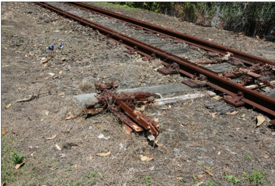
Figure 110: remaining components of railway switch. Weir Phillips
